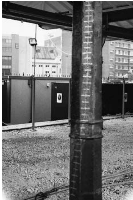
Left: Railway platform support column fractures due to frost and repaired on-site.
